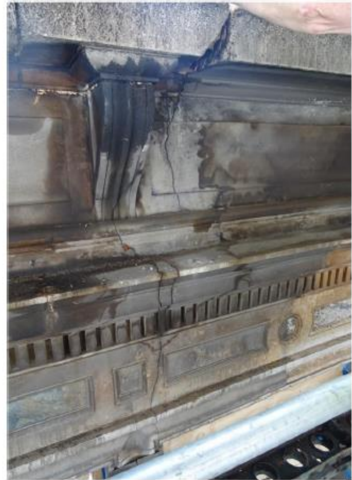
Cracking through all major stone pieces at a structural node in the façade.
