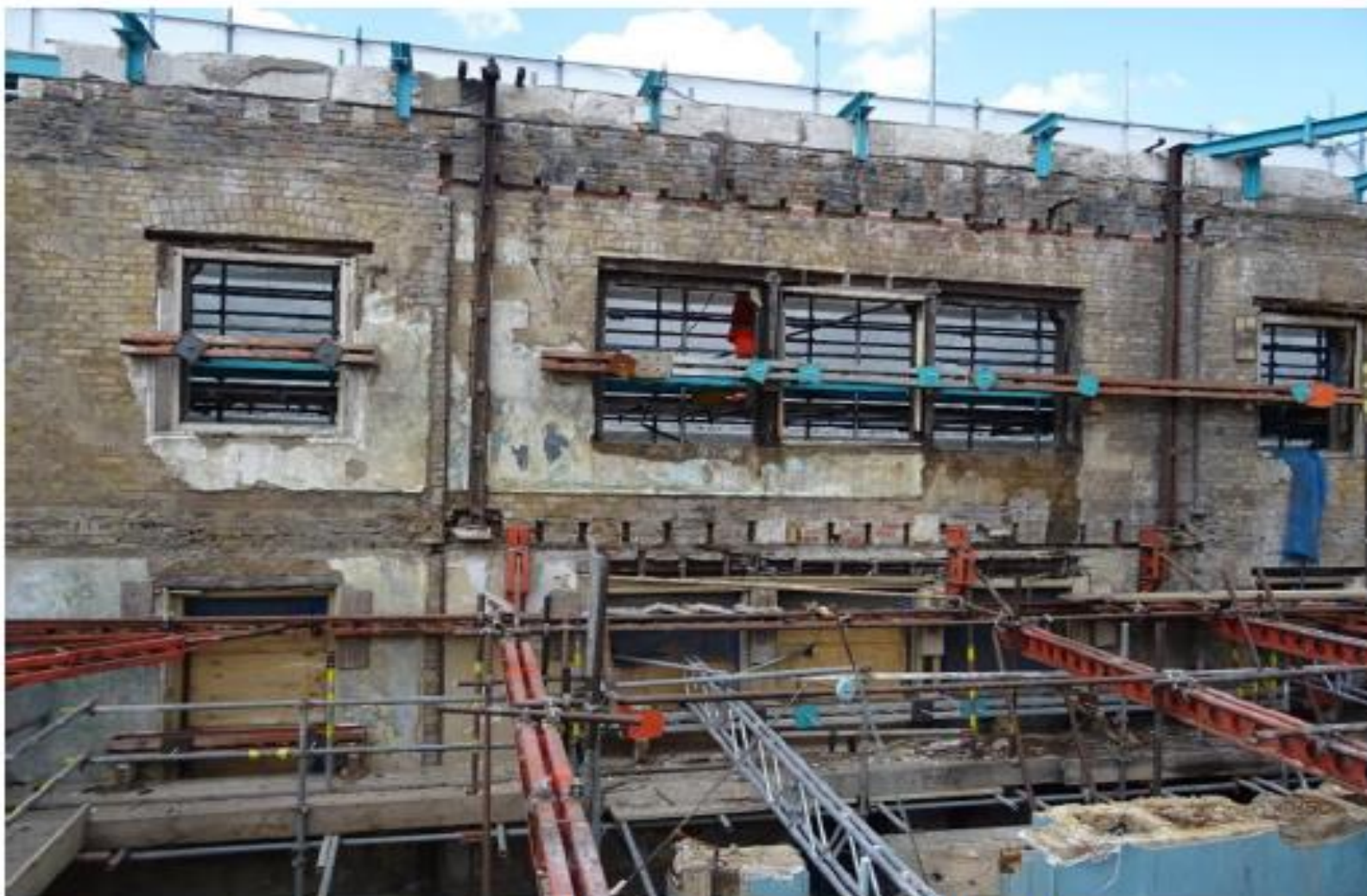
Image showing rear face with decaying brickwork, rotting timber and corroded metalwork.
