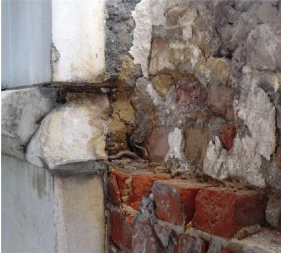
Image showing the poor quality brickwork behind the outer skin of stone.
